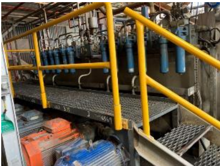
Press Hydraulic Filter Bank
