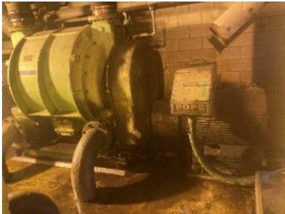
Suction Pick Up #8 and 2 nd Press #9 Vacuum Pumps
