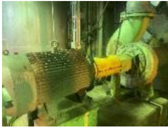
Top Ply Low Pressure Consistency Dilution Pump Motor: POPE, D315S, 415V/75kW/6P Pump: AHLSTROM APP53-250, 170l/s, 26.6m
