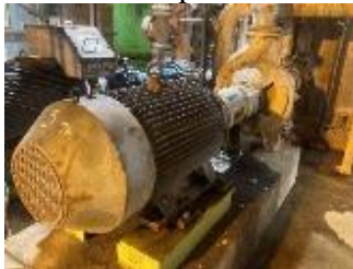
High Pressure Fresh Water Shower Primer Pump 816-30-57 Motor: POPE, D280M, 415V/37kW/4P Pump: AHLSTROM APP33-125
