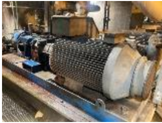
Low Pressure Fresh Water Shower Pump 816-30-141 Motor: POPE, D315M, 415V/132kW/6P Pump: AHLSTROM APP55-200, 114.2l/s, 51.7m
