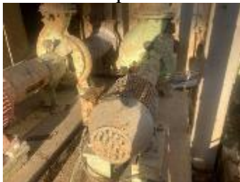
Base Ply HP Consistency Dilution Pump Motor: POPE, D315M, 415V/132kW/4P Pump: AHLSTROM APP53-100, 108.3l/s, 69.1m
