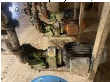
PM6 Machine Hydraulics Cooling Pump 816-30-381 Motor: POPE, D160M, 415V/11kW/2P Pump: AHLSTROM APP22-32, 200l/min, 340kPa
