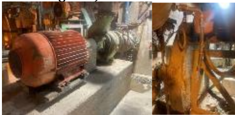
Base Ply White Water Silo Pump
