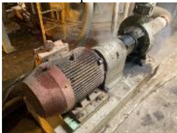
Fresh/Bore Water Booster Pumps x 3 Motor: POPE, D160L, 415V/18.5kW/2P Pump: AJAX 2L, 120GPM 220ft
