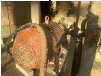
Top Ply Cleaner Dilution Supply Motor: POPE, D200L, 415V/18.5kW/6P Pump: AHLSTROM APP41-300, 158.3l/s, 8.1m
